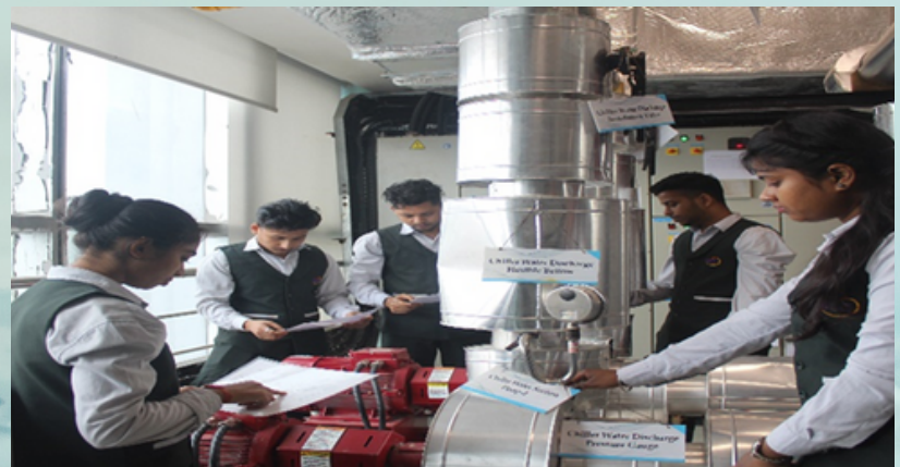
Integrated Building Management Systems Lab
